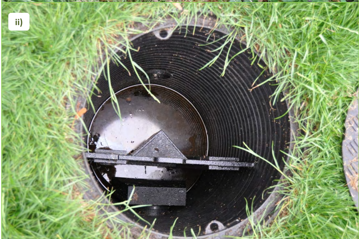
Figure 33. Images from the storm simulation event at Beatrice House swale, Queen Caroline Estate, 29th July 2016. Images show that no water was released to the i) swale overflow or ii) the control flow chamber, after the 10,000 Litres of water were pumped into the swale to simulate a 1 in 100 year storm event.
