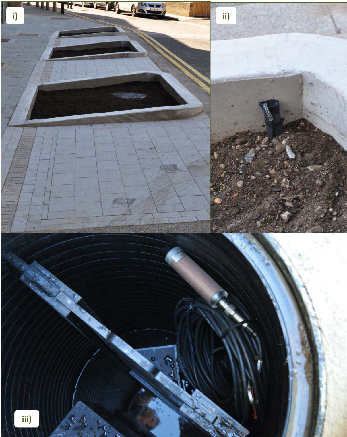
Figure 38. Images from the storm simulation event at the Sun Road rain gardens, Cheeseman Terrace Estate, 23rd September 2016. Images show i) Cheeseman Terrace Estate rain gardens before rain simulation; ii) pressure sensor installed in the corner of one of the rain gardens; iii) pressure sensor installed in the control flow chamber in the outlet from the rain garden.
