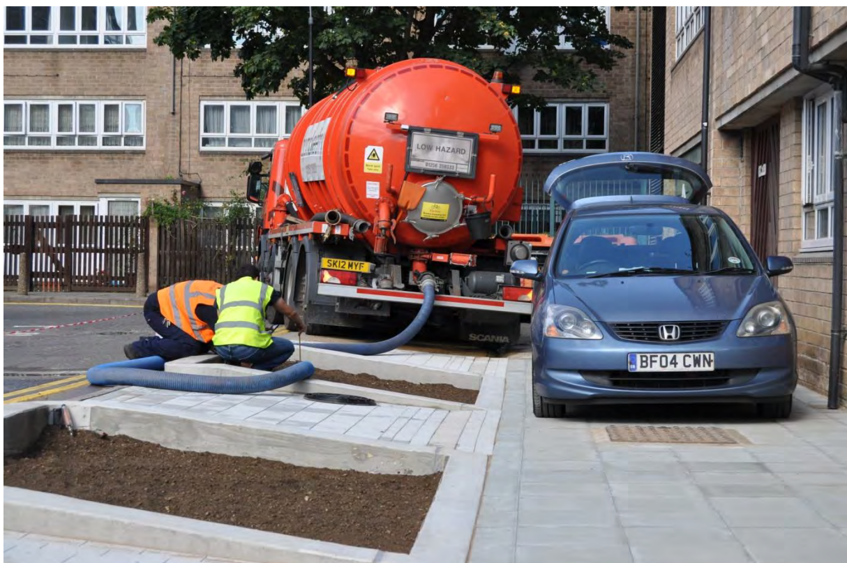
Figure 36. Water tanker delivering 6000 Litres of non-potable water for the storm simulation event at Cheeseman Terrace Estate. Storm simulation was carried out over the course of an hour on the 23rd September 2016.
