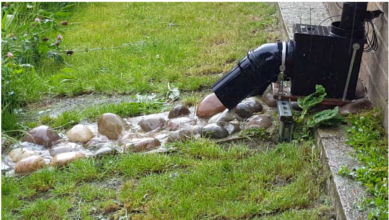
Figure 28. Beatrice House downpipe outflow. Image shows runoff from downpipe to ground level swale during a storm event on the 16th June 2016.
