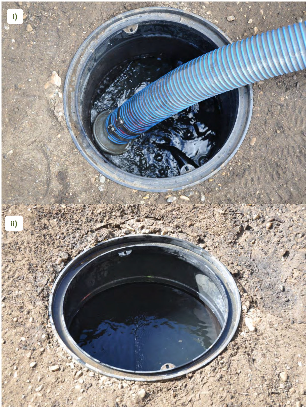
Figure 39. Images from the storm simulation event at the Sun Road rain gardens, Cheeseman Terrace Estate, 23rd September 2016. Images show i) water being pumped into the inspection chamber of the rain garden; ii) inlet chamber full after the stormwater was pumped in.
