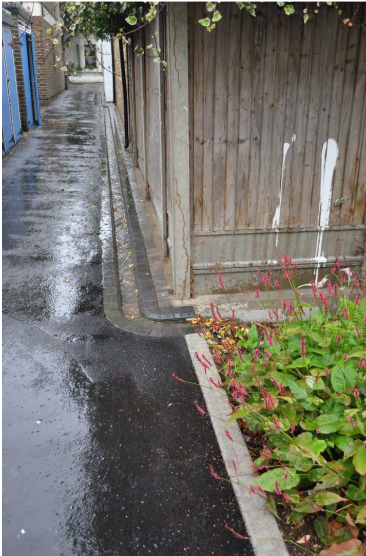
Figure 38. Water from roof level and ground-level hard standing being channelled into the rain garden at Richard Knight House during a heavy rain event on the 24th August 2015.
