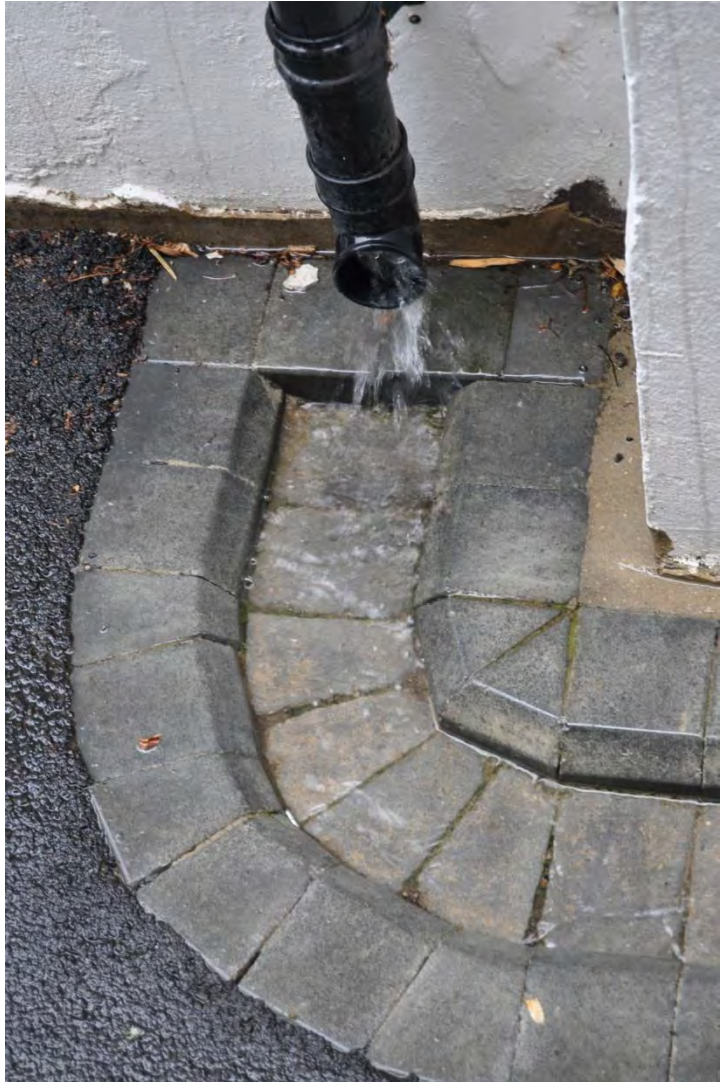
Figure 36. Water being channelled from roof level to the rain garden at Richard Knight House during a heavy rain event on the 24th August 2015.
